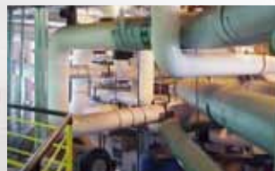
33RD STREET JAIL MECHANICAL SYSTEMS
