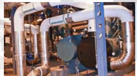
KINGS BAY THERMAL CHILLER
