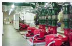
FEDERAL LAW ENFORCEMENT CHILLED WATER SYSTEM
