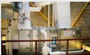
NAS JAX HANGAR 1000 CENTRAL ENERGY PLANT
