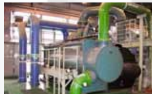
JOHNSON SPACE CENTER CHILLER SYSTEMS
