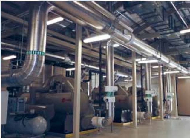
KEESLER MEDICAL CENTER CENTRAL ENERGY PLANT
